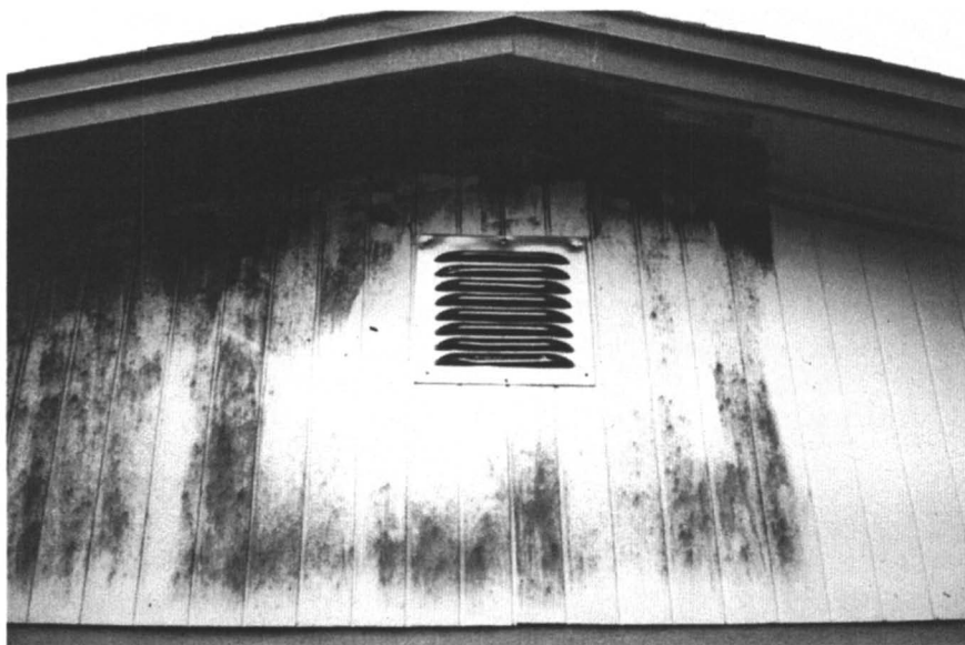
Figure 1. Black mold on a gable in New Jersey. The portion to the right has been cleaned.
