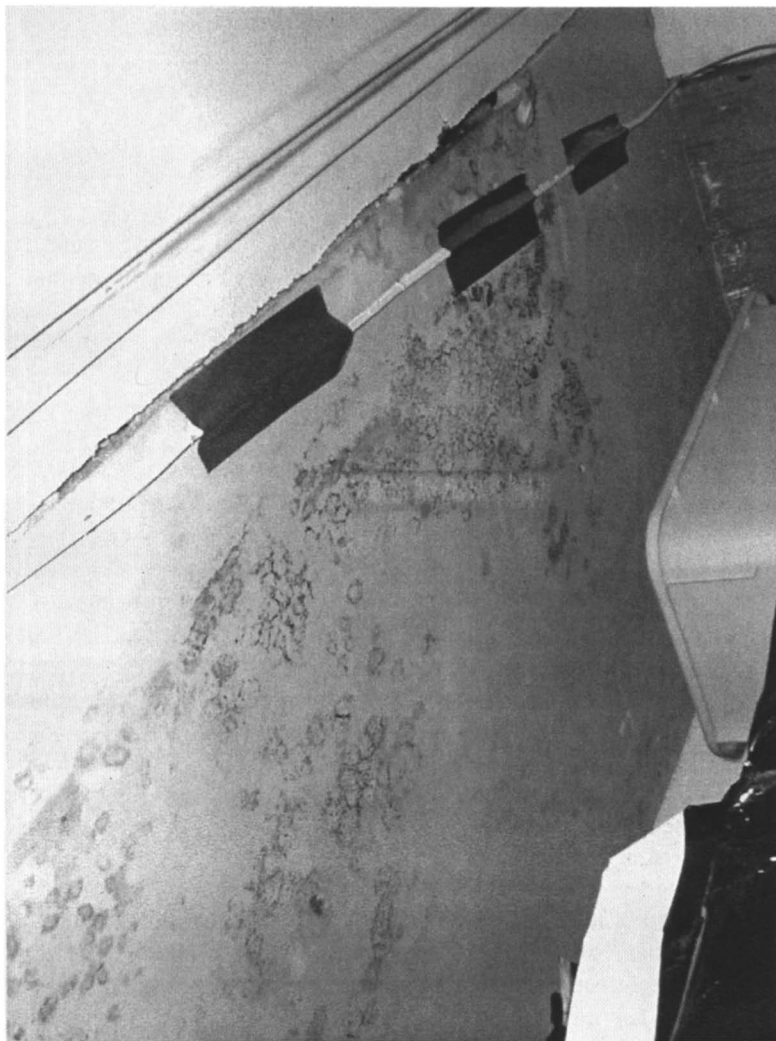
Figure 1. Stachybotrys atra growing on gypsum wall board. The source of water was a leak at the deck to wall interface located above this ceiling space.
