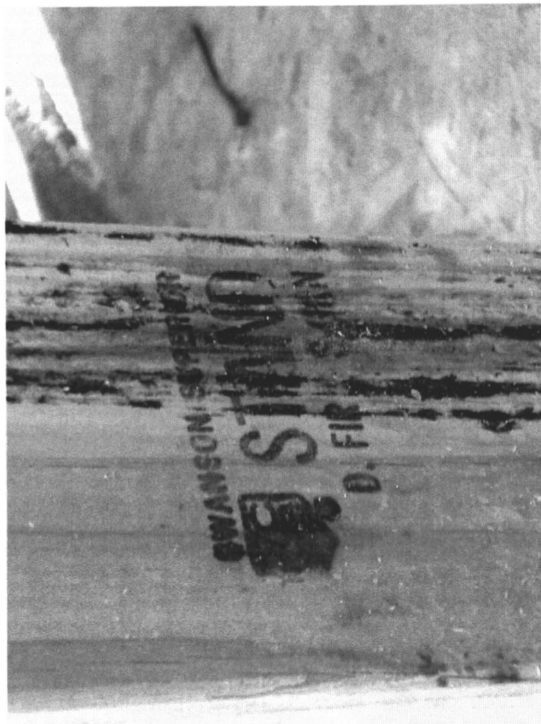
Figure 2. The use of non-kiln dried ('green') lumber in construction in California and other portions of the western United States has resulted fungal growth being 'built in' in many buildings. Note the abrupt transition in fungal growth on this stud, coinciding with the transition from sapwood (fungal growth) to heartwood (no fungal growth).
